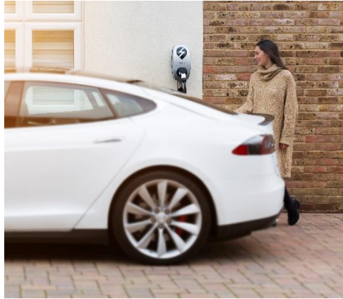
Charge point & electricity connection installed
